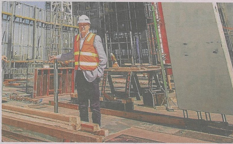
Multiplex regional managing director Graham Cottam on site at the Collins Arch project last week where "spalling" has occurred. PHOTO: EAMON GALLAGHER
